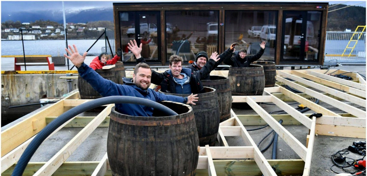
Figure: The youth building a temporary structure, supervised by the contractors, Credit: Memoria (upper) and Bypatrioten (lower)
