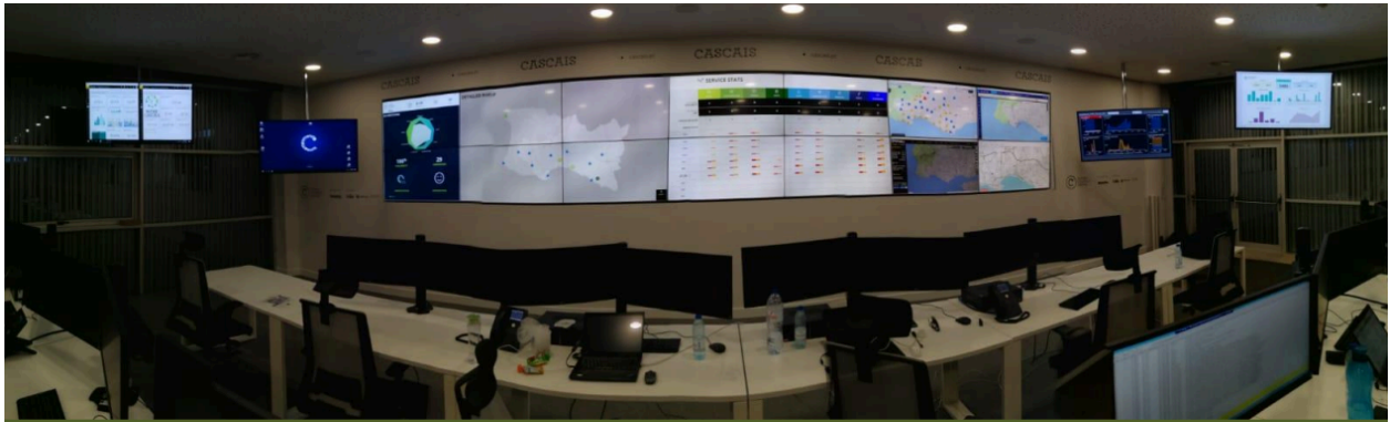
Figure 38: Cascais control centre 22 .
