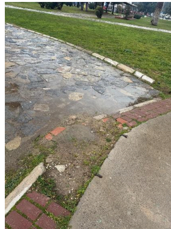
Figure 13: Potholes in the area
